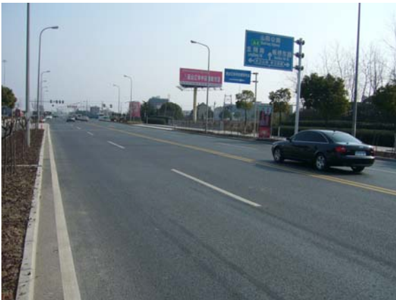
Fig. 9 Pavement Conditions for KimShan Broadway After 1 year of Trafficking
