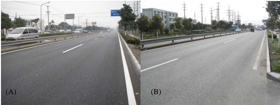
Fig. 6 Pavement Conditions for Huchinping Highway After (A) 1 Month and (B) 2 Years of Trafficking
