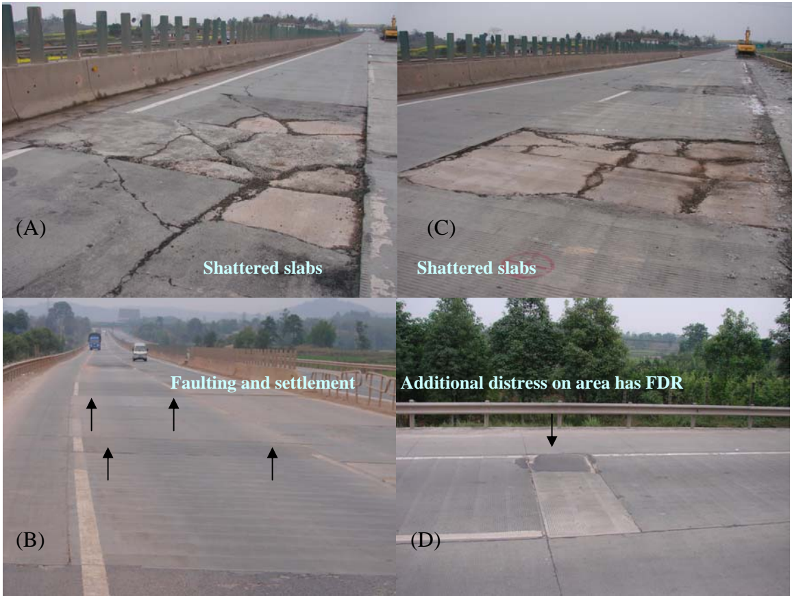
Fig. 2 Severe Distresses Including (A &B) Shattered Slabs, (C) Faulting/ Settlement (D) Additional Distress Reappeared on Area where received Full Depth Repair (FDR)
