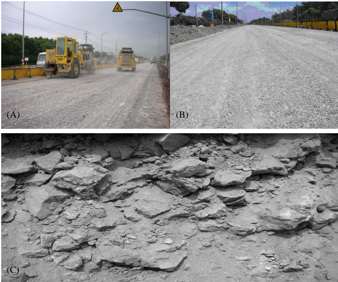
Fig. 5 Rubblization Using Resonant Breaker on Huchinping Highway (A) Two RMI RB500 Resonant Breaker in Action (B) Rubblized Surface Condition Before Rolling, and (C) Test Trench Show Fractured Particles Throughout Entire JCP Thickness.
